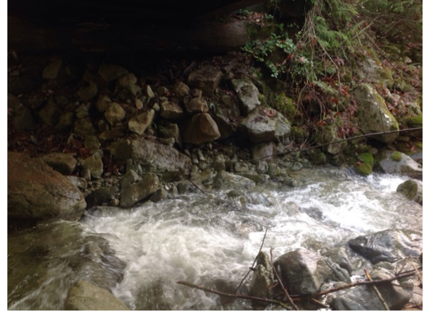
left bank D/S riprap scour
